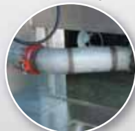
Stainless steel plumbing
