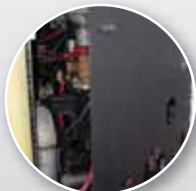
Hinged pump panels
