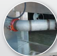
Stainless steel plumbing
